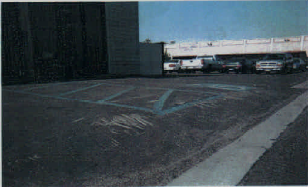
Figure 1 - View of Mental Health parking lot showing slope and grooves in the pavement (11/27/01)
