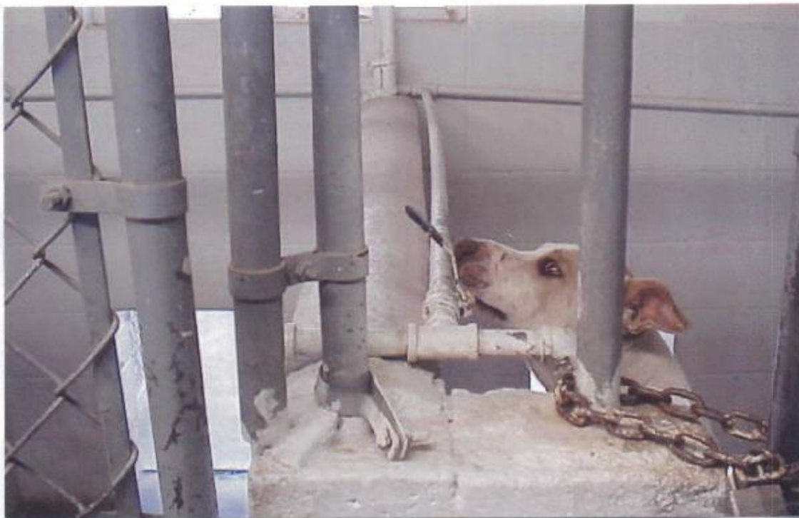
Photograph #3 - Missing upper fencing on kennel that would prevent larger dogs from jumping into another kennel.
