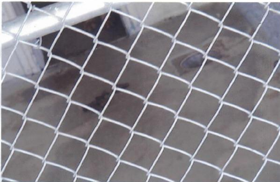
Photograph #5 - Drain holes (6-8" in diameter) in the kennel floor were uncovered.
