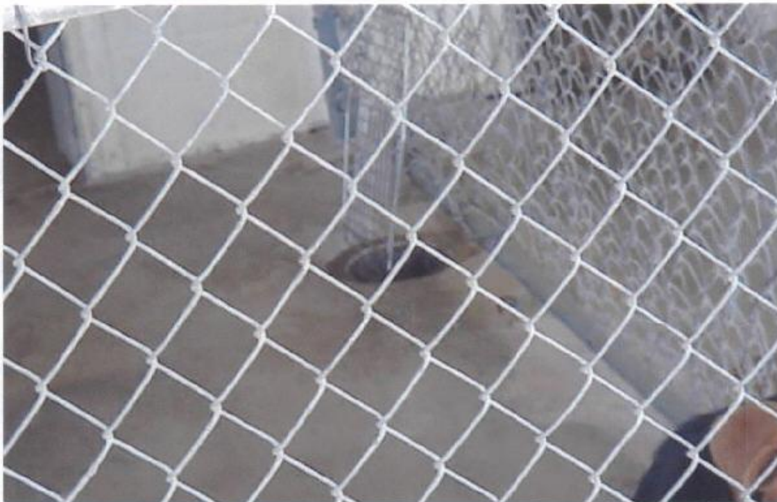
Photograph #4 - Drain holes (6-8" in diameter) in the kennel floor were uncovered.
